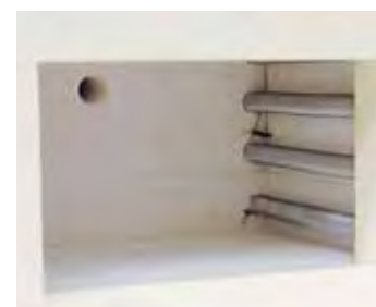
Furnace lining with high-quality lightweight refractory brick insulation
